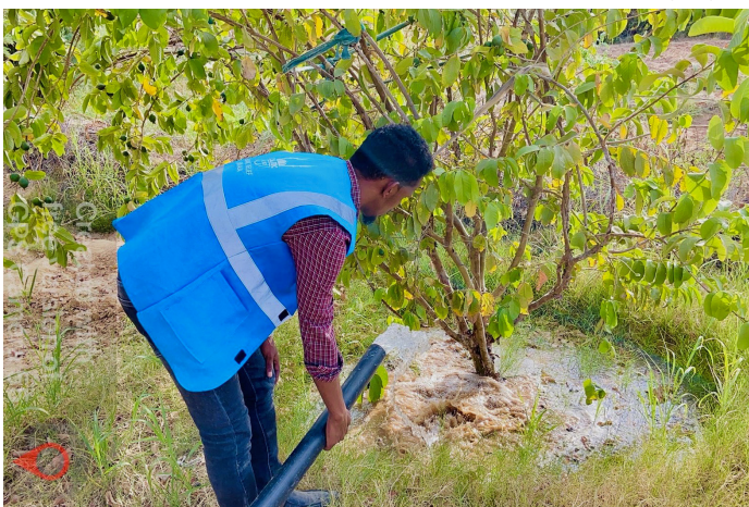
IR staff checking irrigation pipe during the rehabilitation of shallows well in Mindhicir village of Sanag region
