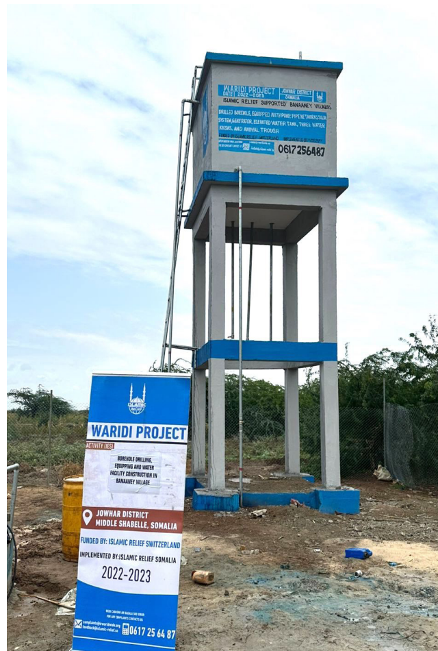
Drilling and equipping of a new borehole in Jowhar district, Middle Shabelle region, Somalia
