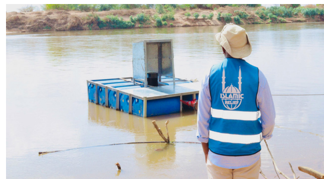
Pipeline extension from the Juba River in Bardhere district to the IDP camps outside Bardhere town, Gedo region, Somalia.
