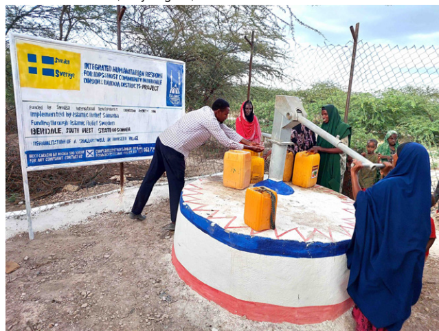
Rehabilitation of 2 shallow wells for the droughts affected families in Berdale district, Bay region, Somalia
